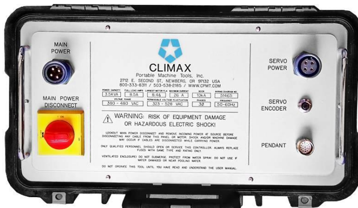
FIGURE 21. SERVO MOTOR CONTROL PANEL
